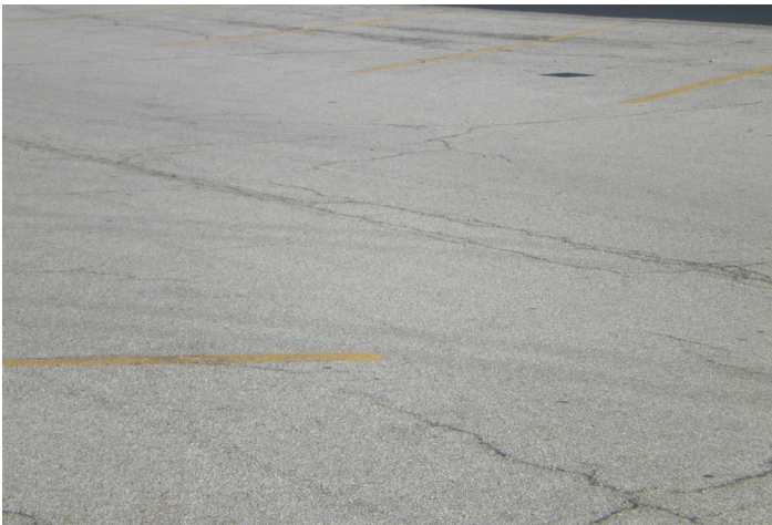
PROBLEM Excessive cracking in existing pavement
