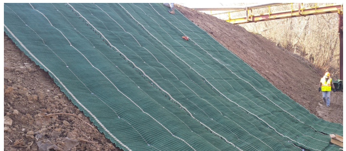
SOLUTION ARMORMAX® was used to repair current damage as well as protect from further erosion
