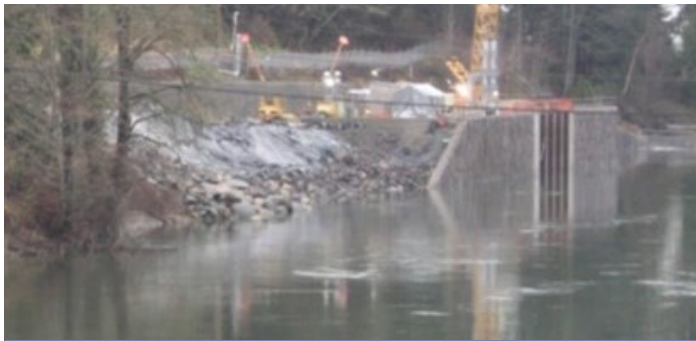
PROBLEM Erosion and slope instability along the Snoqualmie
