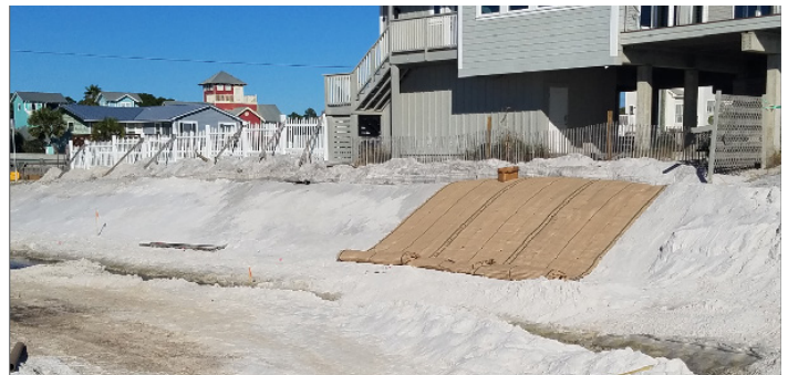
SOLUTION More than 2,000 square yards of ARMORMAX was installed along the outfall
