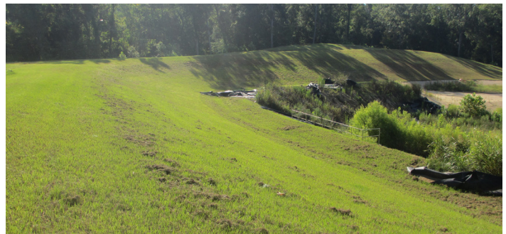
PERFORMANCE The installation is fully vegetated and maintains its integrity despite heavy equipment traffic from regular mowing
