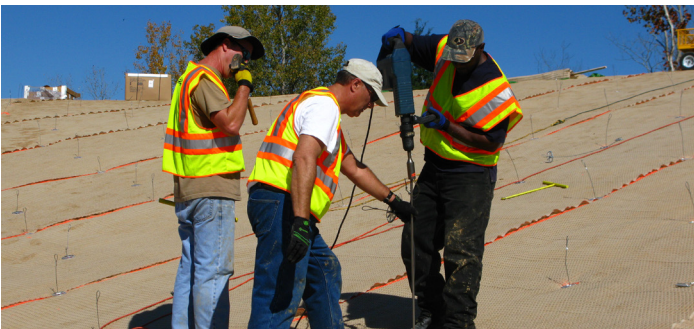
INSTALLATION More than 5,000 square yards of ARMORMAX was installed in just 2 days
